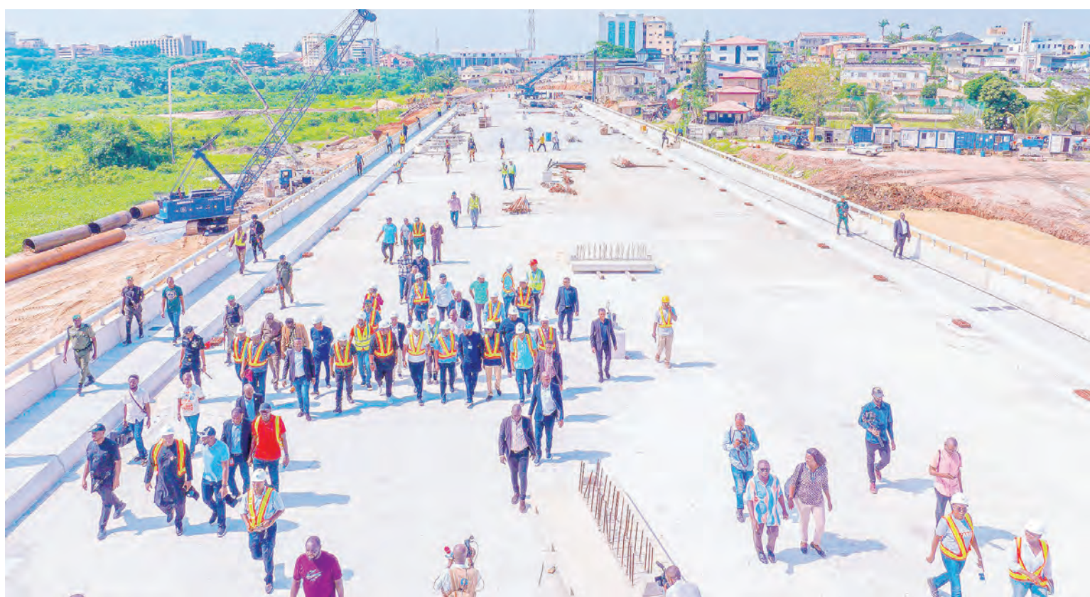
An aerial photograph of the ongoing Opebi-Mende-Ojota Link Bridge in Lagos State.
