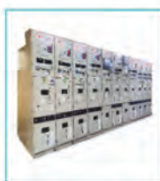
Indoor MV 11kV Switchgear Panel Board
